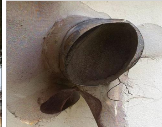
Net on ventilation pipe to prevent insects entering
